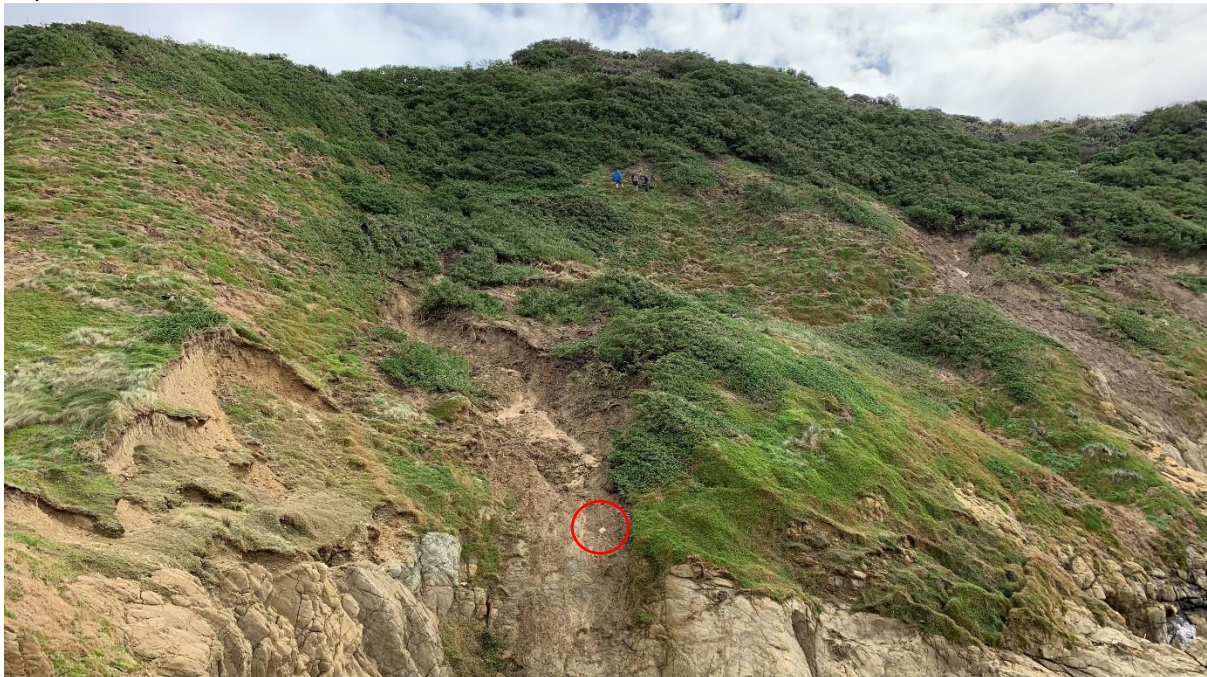
Figure 1 Damage to the pakahā colony at the northern tip on Kokomohua/Long Island after the winter storms in 2022. Note previous slip damage from a few years ago on the lower left-hand side, showing how fragile this site is. Red circle showing an artificial burrow hatch lid from the slip.
